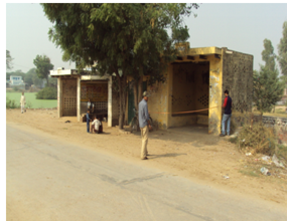
A bus shelter that will have to be rebuilt
