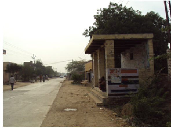
A bus shelter that will have to be rebuilt
